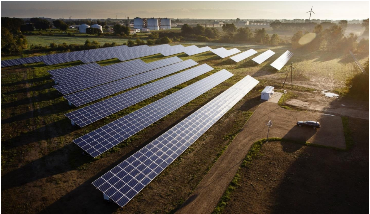
Photovoltaic farm in Bystra
