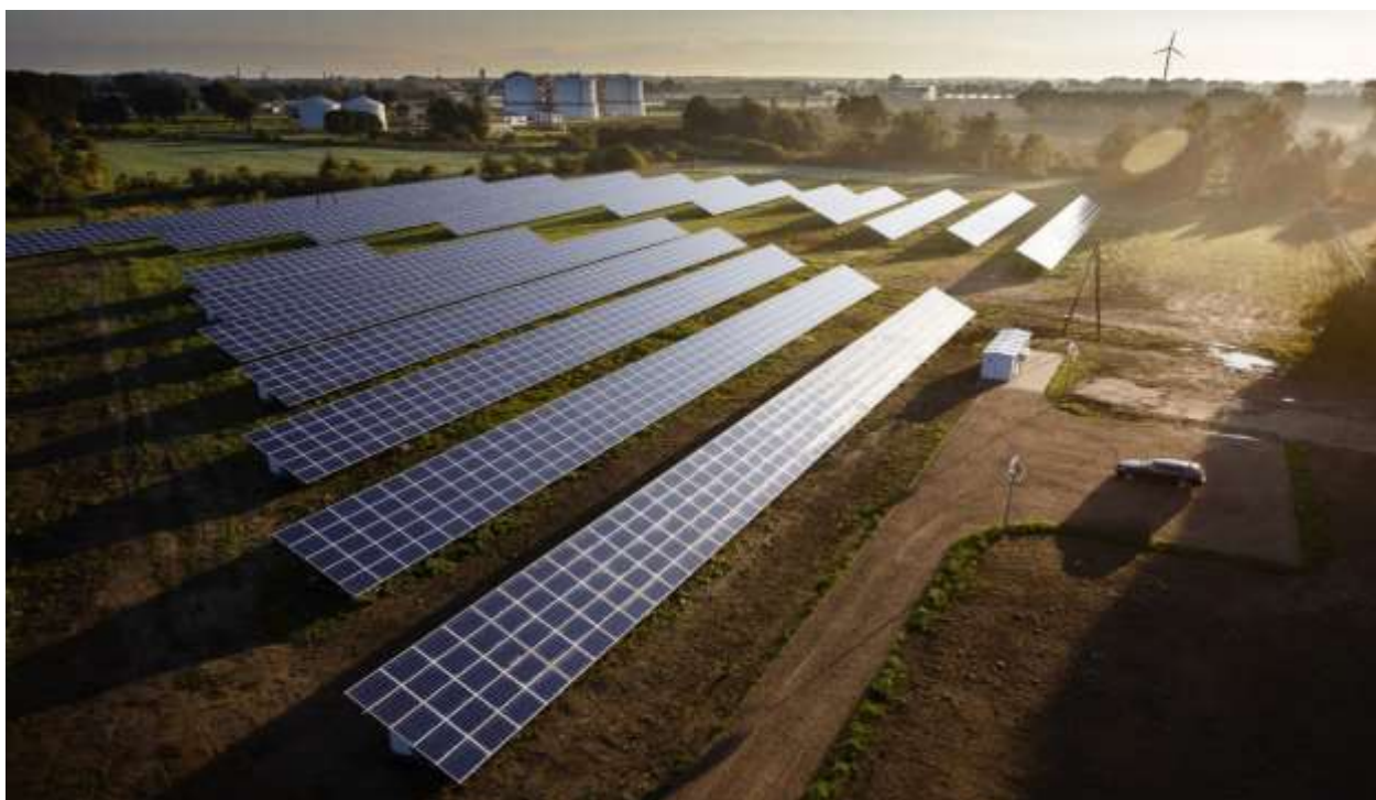
Photovoltaic farm in Bystra
