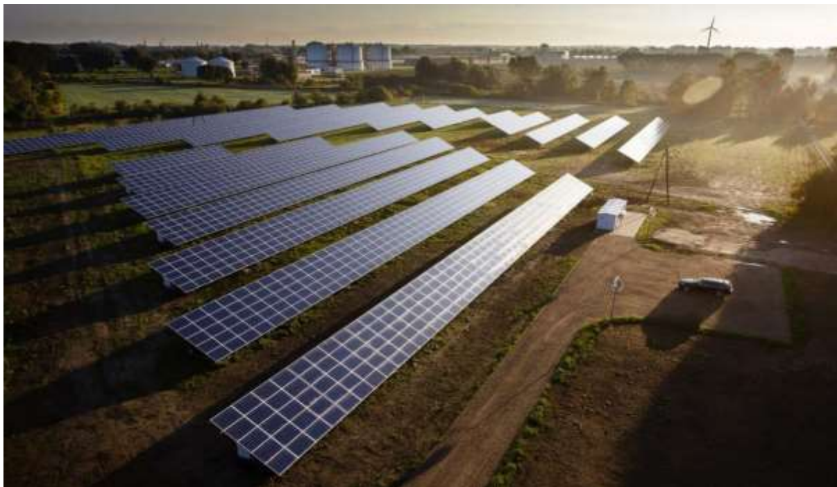
Photovoltaic farm in Bystra
