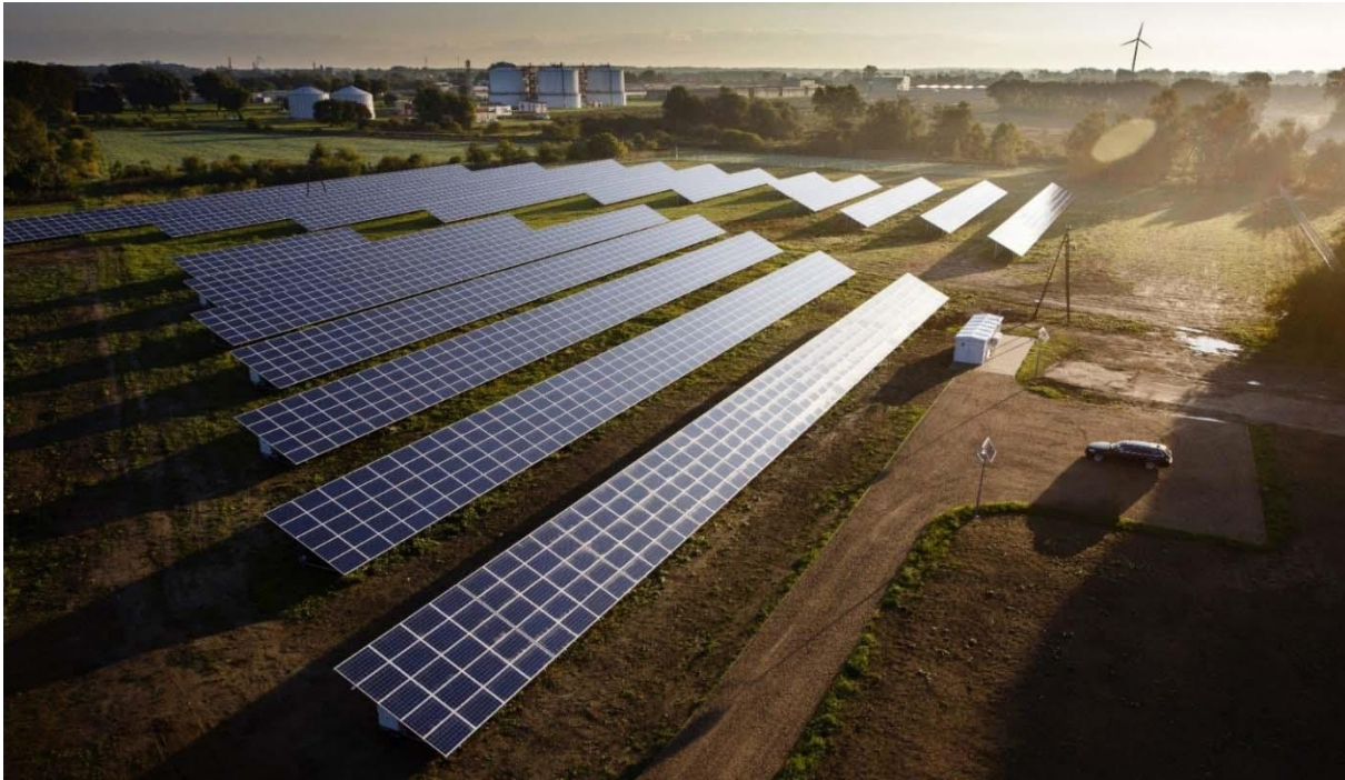
Photovoltaic farm – Bystra, municipality of Gdańsk
