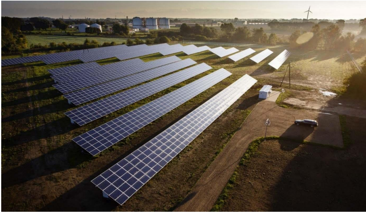
Photovoltaic farm in Bystra
